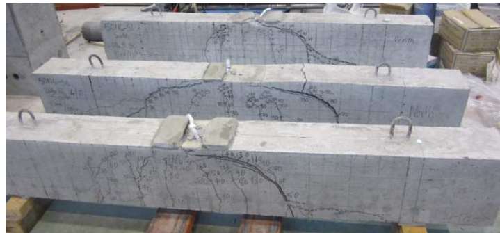
Photo 2. Overall view of cracked RC beams
